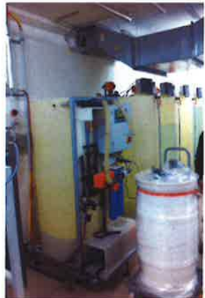
Bulk acid storage tanks
